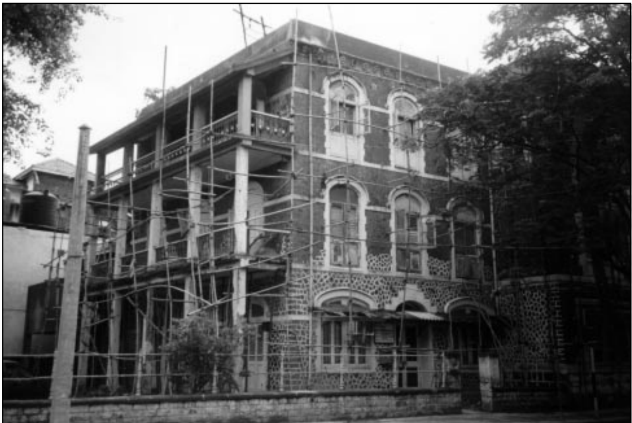
Figure 50 Older building in Mumbai undergoing nonseismic-related repair and maintenance due to problems with corrosion.
